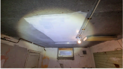
Plater i himlingen inneholder asbest
