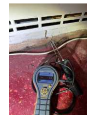
Gammel fuktskade under aggregat.
